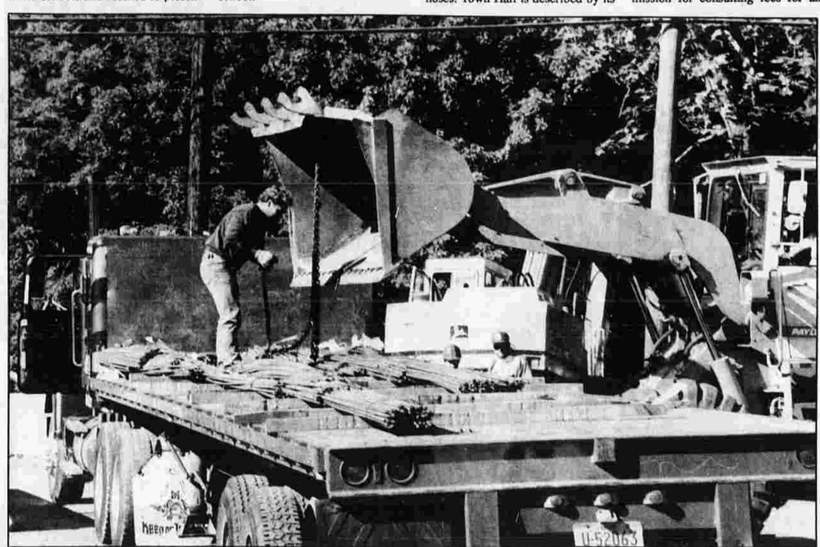
HEAVY CONSTRUCTION — Rick Osgood of East Hartford works on a water and sewer construction project on Highland and Oak Grove Streets in Manchester. He works for Central Paving Inc. of South Windsor.
